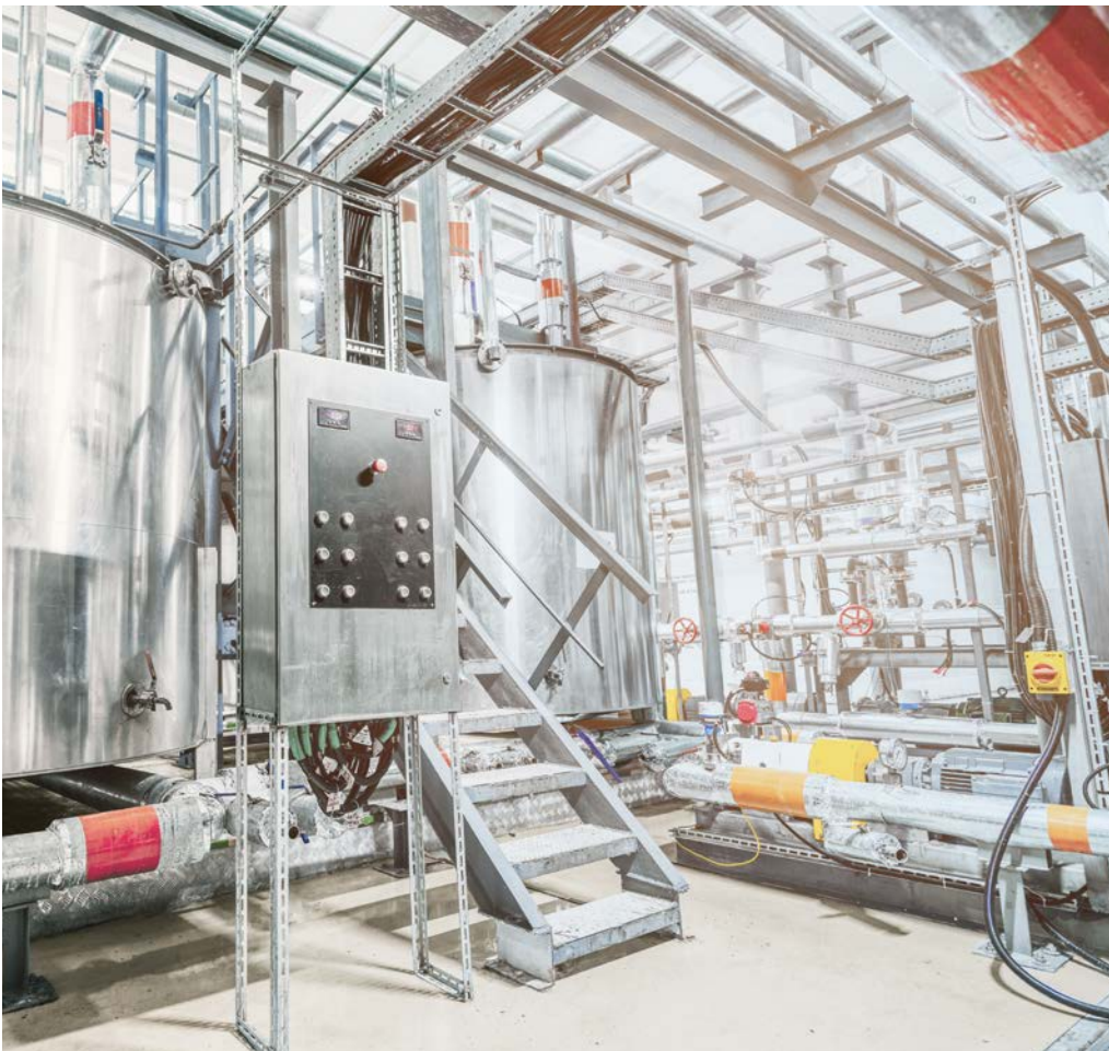
Industrial plants such as these must be anchored according to the standards of the facilities regulation (AwSV).
